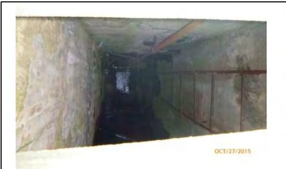
Photo 24 – Photo from previous Tighe & Bond inspection, taken on 10/27/15 showing interior of low-level outlet's intake structure and gate valve; note minor leakage, ladder constructed of rebar, gate stem appears bent
