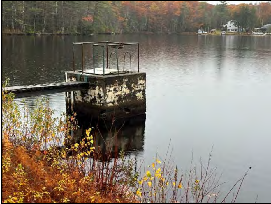
Photo 27 – Left side of intake structure; note spalls and concrete erosion, especially near water line (Photo taken by Tighe and Bond on 10-30-23)
