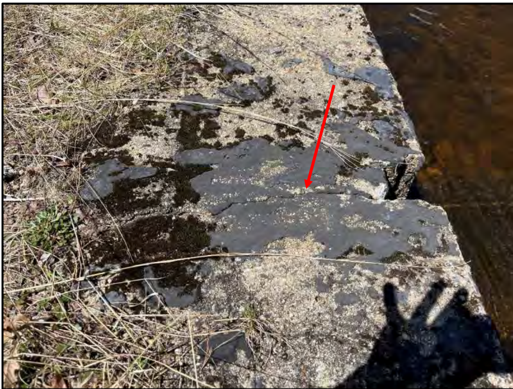
Photo 20 – Transverse crack in right training wall at the flashboard slot
