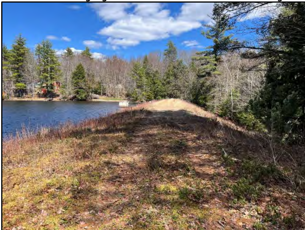
Photo 2 – Overview of dam crest from right abutment; note trees within 20 feet of embankment and minor rutting (tire tracks)
