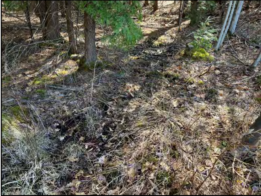
Photo 5 – Wet area at downstream toe near right abutment
