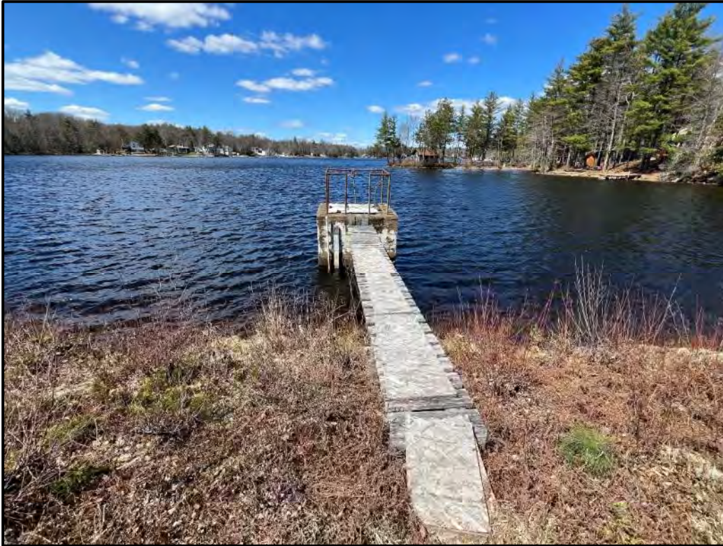
Photo 1 - Overview of impoundment and low-level outlet structure; note mounted staff gauge and absence of handrails on footbridge
