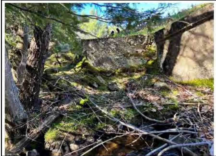
Photo 23 – Photo from previous Tighe & Bond inspection, taken on 5/11/22 showing downstream section of right training wall with concrete deterioration and vegetation near the wall
