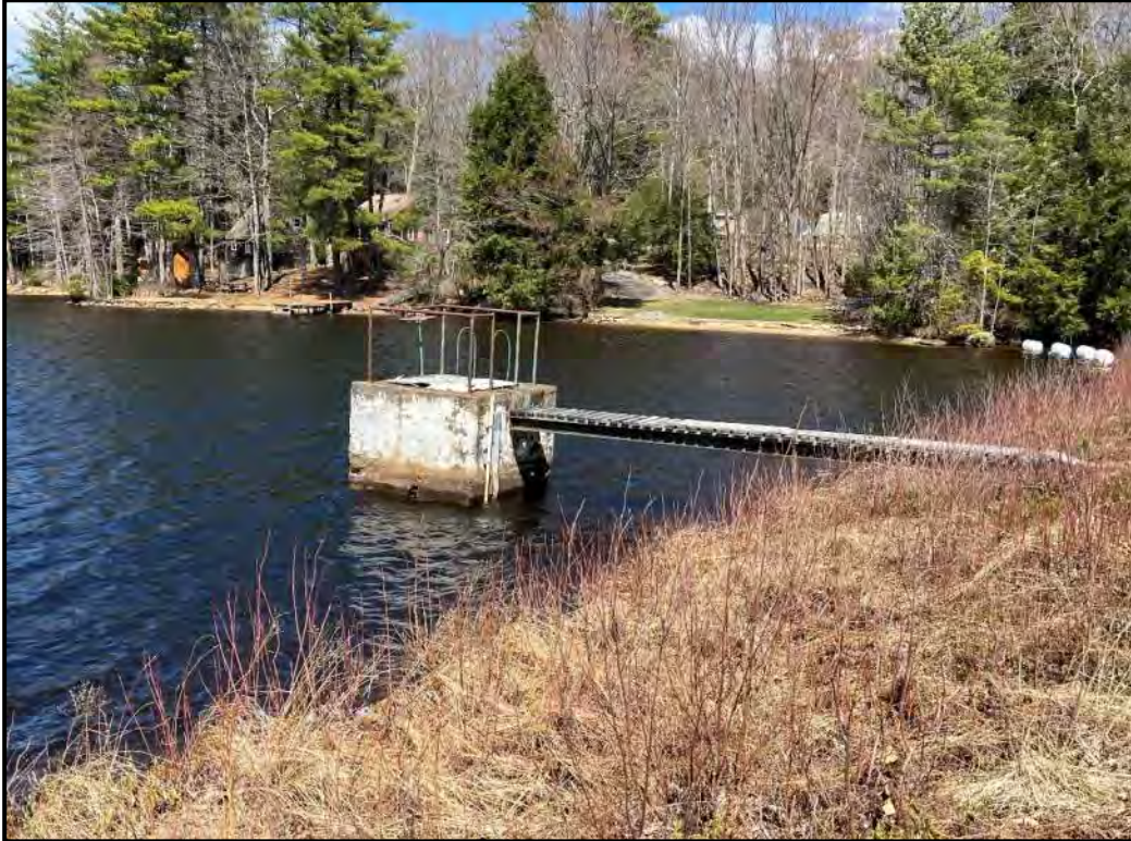
Photo 13 – Right side of intake structure; note spalls and concrete erosion; see Photo 26 from Oct 2023 with lower reservoir level
