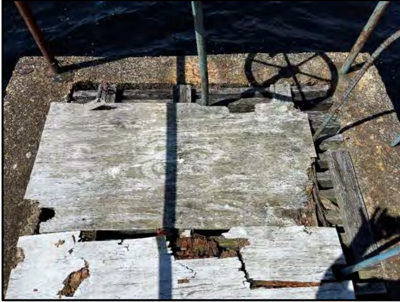
Photo 15 – Top of low-level intake structure. Wood grating and deteriorating plywood boards partially obscured interior of structure
