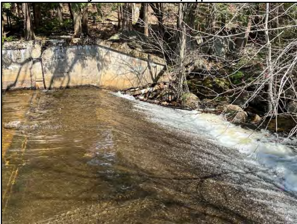
Photo 18 – Left spillway training wall; note cracking, efflorescence, and trees growing adjacent to the wall
