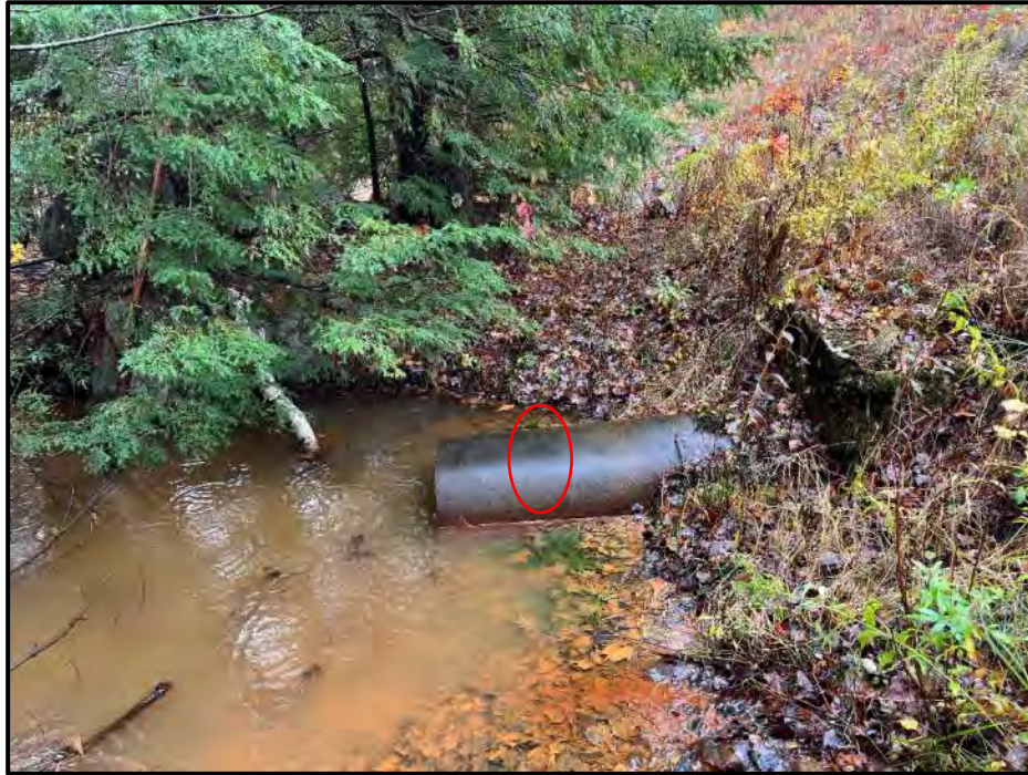
Photo 25 – Outlet structure discharge conduit with crack (Photo taken by Tighe and Bond on 10-30-23)
