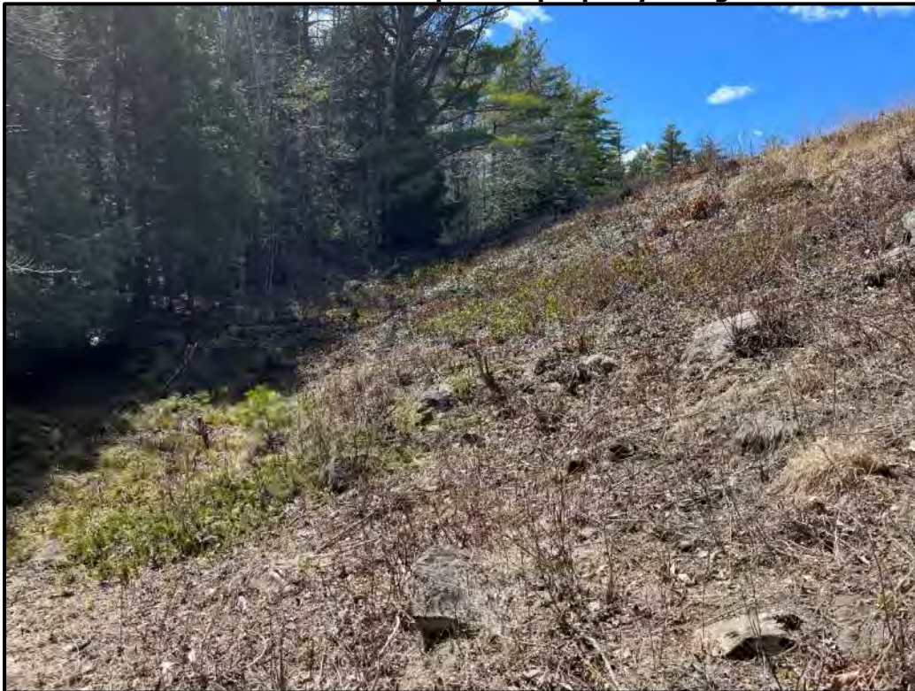
Photo 4 – Downstream slope near right abutment; note cobbles and areas of bare vegetation on slope and trees within 20 feet of dam
