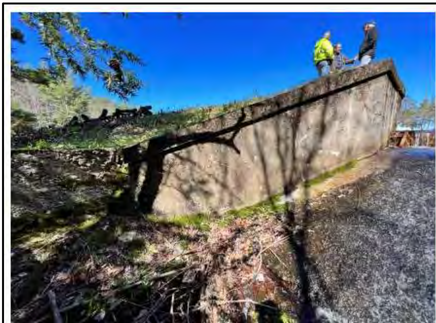
Photo 22 – Photo from previous Tighe & Bond inspection, taken on 5/11/22, showing right training wall with minor cracking and efflorescence
