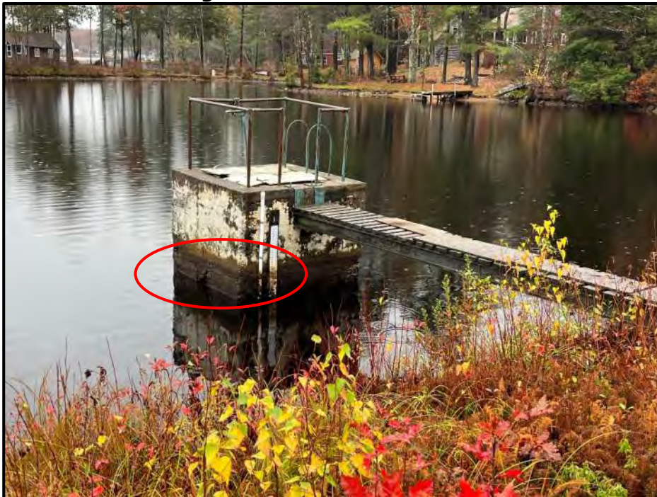
Photo 26 – Right side of intake structure; note spalls and concrete erosion, especially near water line (Photo taken by Tighe and Bond on 10-30-23)
