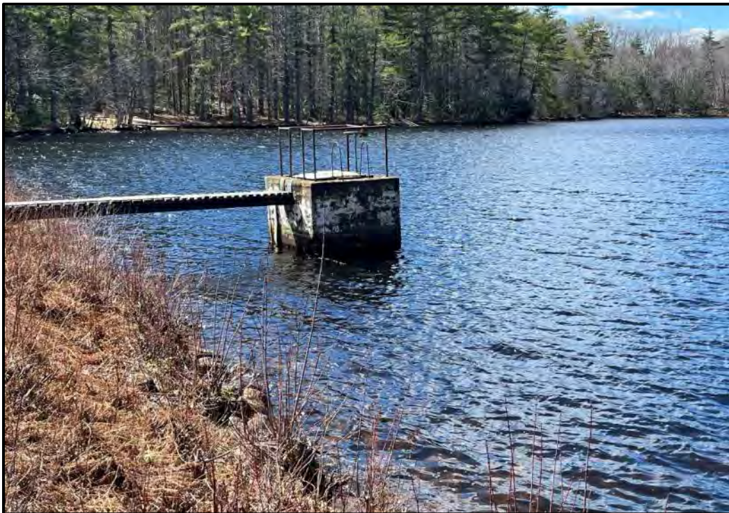
Photo 14 – Left side of intake structure; note spalls and concrete erosion; see Photo 27 from Oct 2023 with lower reservoir level
