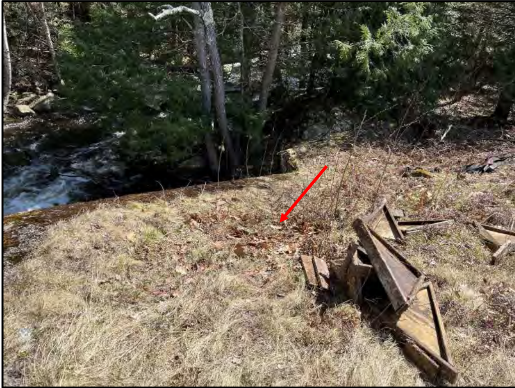
Photo 19 – Downstream embankment behind right spillway training wall; note depression behind wall
